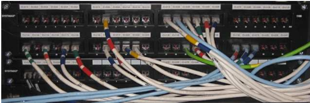
Figure 3. A 72-port patch panel with 60 ports terminating in the cross-connect cabinets.
