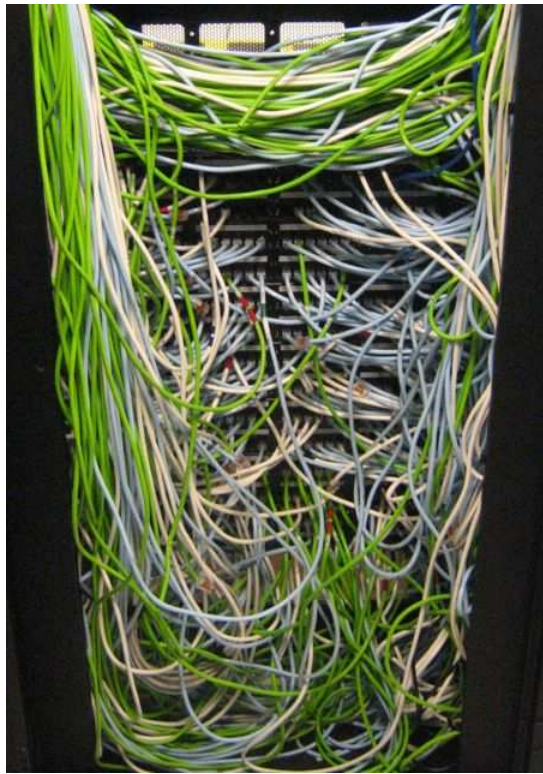
Figure 2. Existing cabling in a cross-connect cabinet in the data centre.
